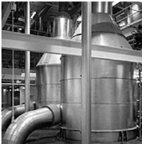
Figure 14.4 Large crystallizers in wastewater treatment. (Courtesy of General Electric)
