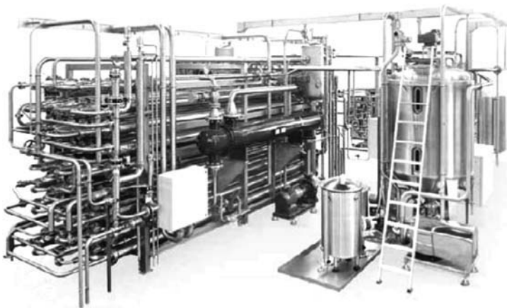
Figure 3.14 Tubular heat exchanger assembly in aseptic processing plant. (Courtesy of Rossi & Catelli)
